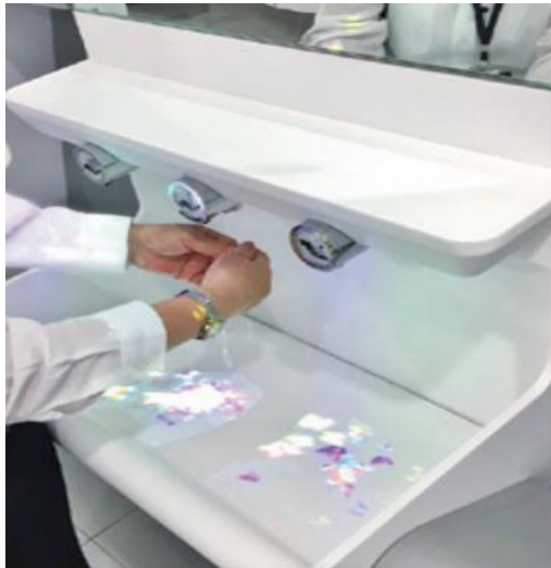
Figure 5.4 "One-stop" Hand-washing and Hand-dryer in One Basin
